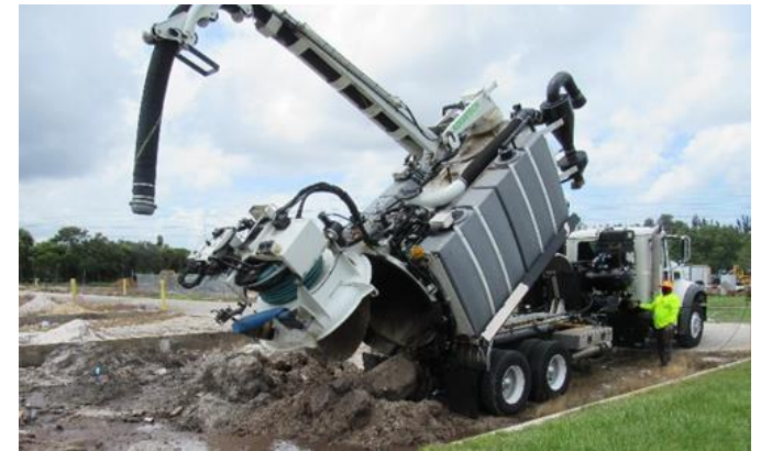
Heavy-Duty Vector Truck for sewer cleaning
