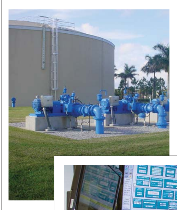
High service pumps Lake Region Water Treatment Plant Belle Glade, FL
